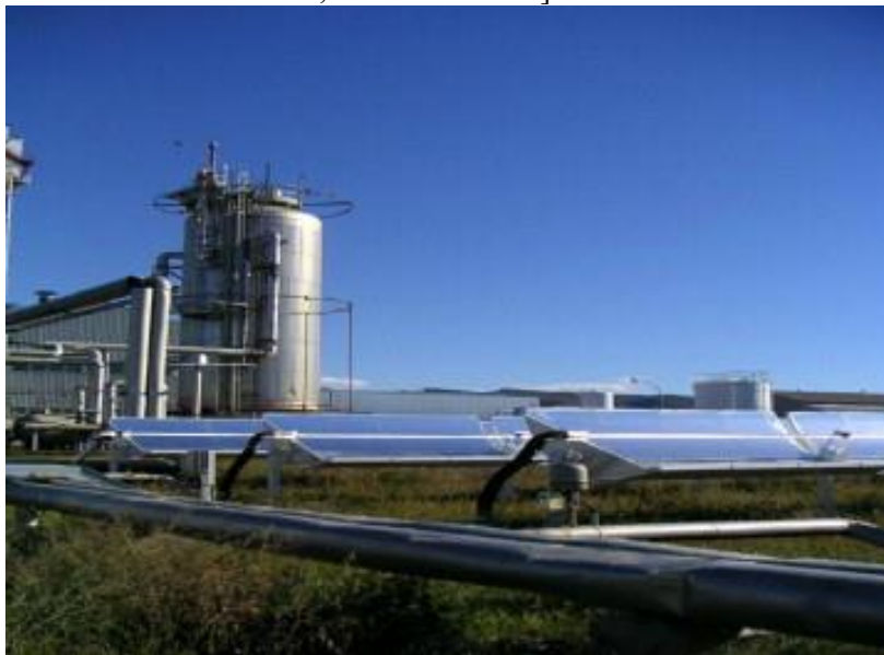
Rys. 1 3 . (Fig. 1. The ACUREX solar field and the thermal storage tank.(p. 3.3.2. praca 1 Reference governor ...)
